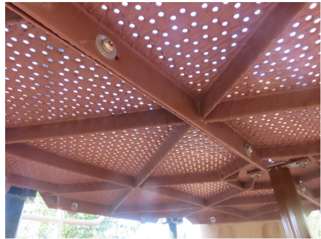
Underside and fasteners of playset in good condition
