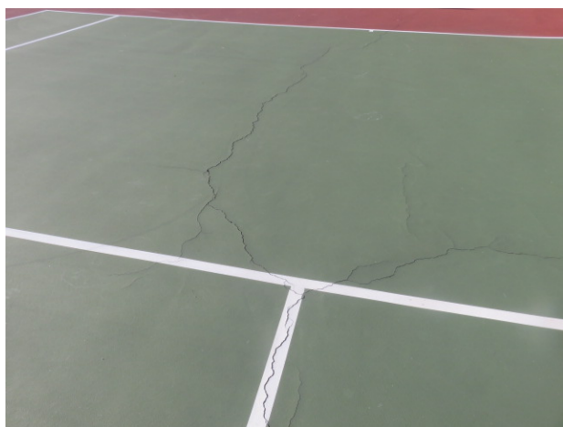
Surface cracks at tennis court
