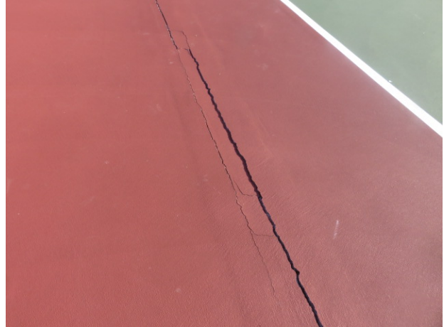
Cracks at tennis court surface
