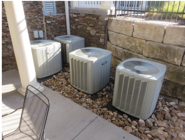
Clubhouse condensing units
