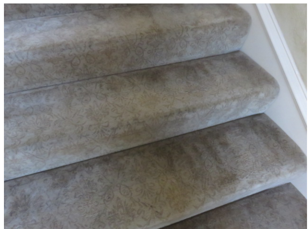
Carpet wear at staircase
