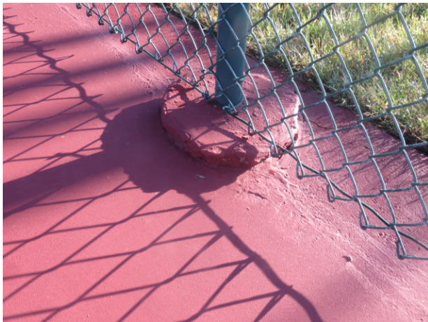
Settlement of asphalt below concrete fence footing
