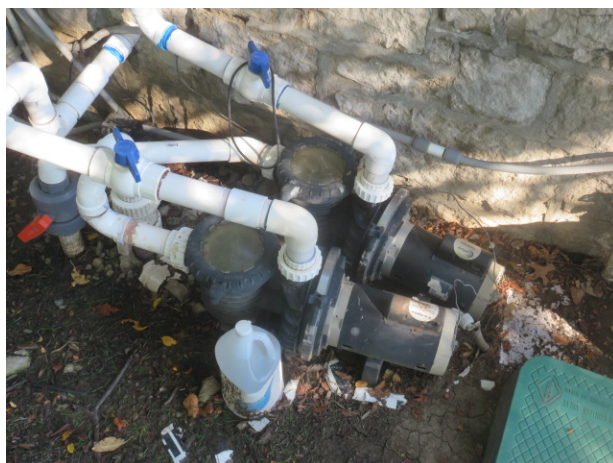
Fountain mechanical equipment
