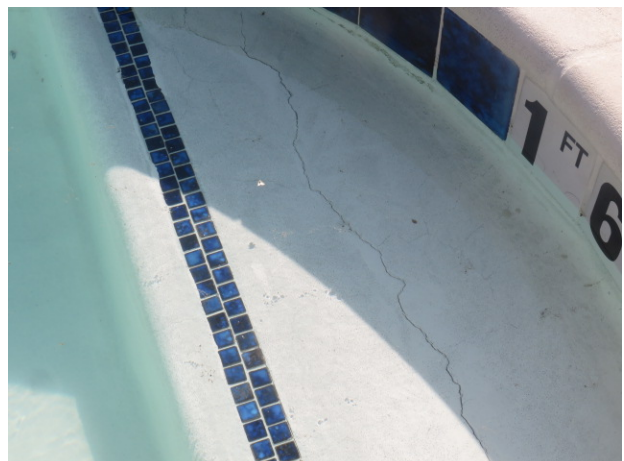
Large crack at wading pool step
