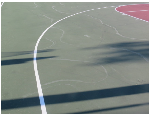
Evidence of previous standing water at basketball court
