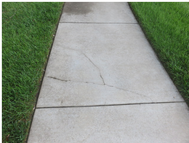
Isolated and minor sidewalk cracks
