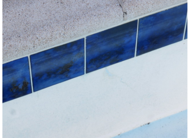
Plaster finish deterioration
