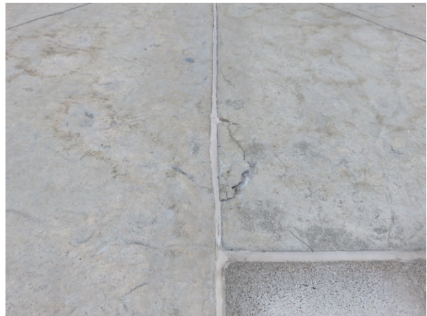
Isolated "D-crack" along control joint
