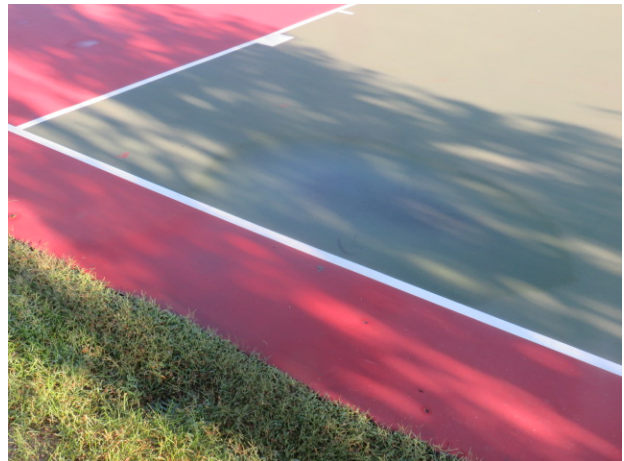
Settlement and minor instance of standing water at basketball court
