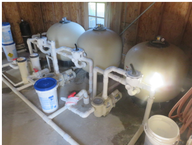
Pool pumps and filters
