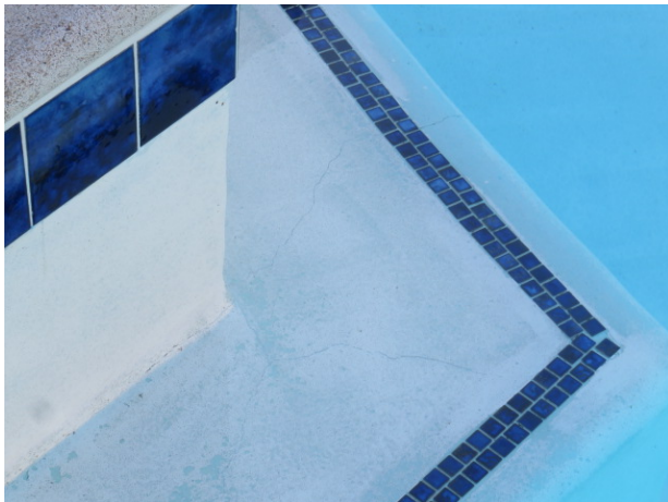
Minor cracks at pool shelf
